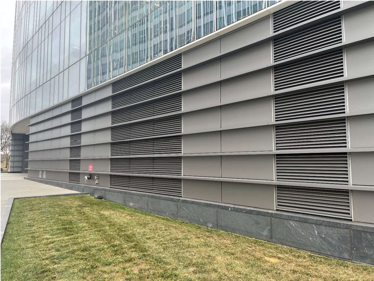
Ground Floor Mechanical Room Intake (center) & Exhaust (Left & Right)
