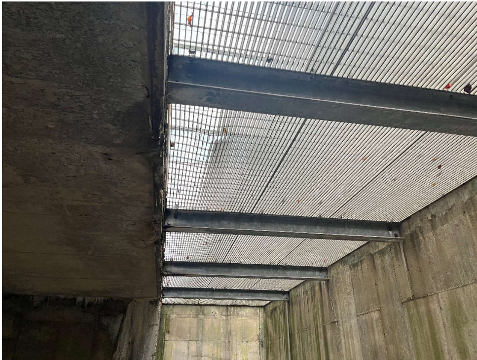
Fresh Air Intake for all ground floor Mechanical systems
